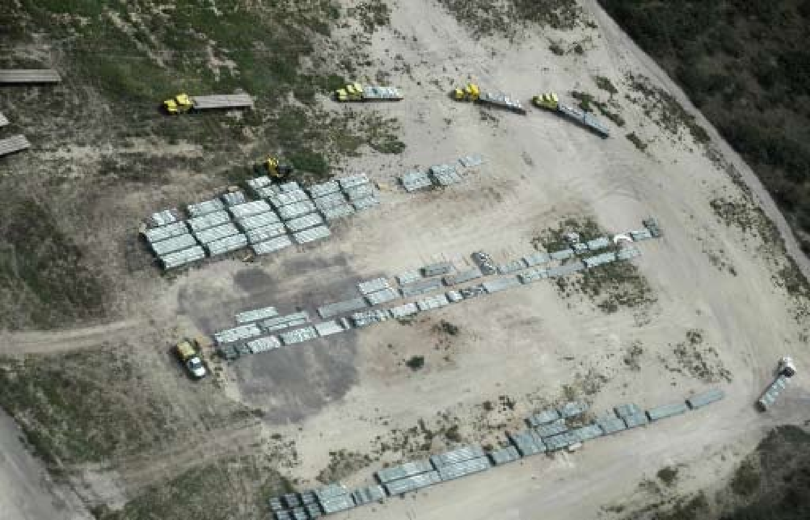
LCRA rented a temporary laydown yard, approx. 40 acres, near Junction, TX. Yellow delivery trucks from Mexico stock pile loads of steel lattice tower materials July, 2010
