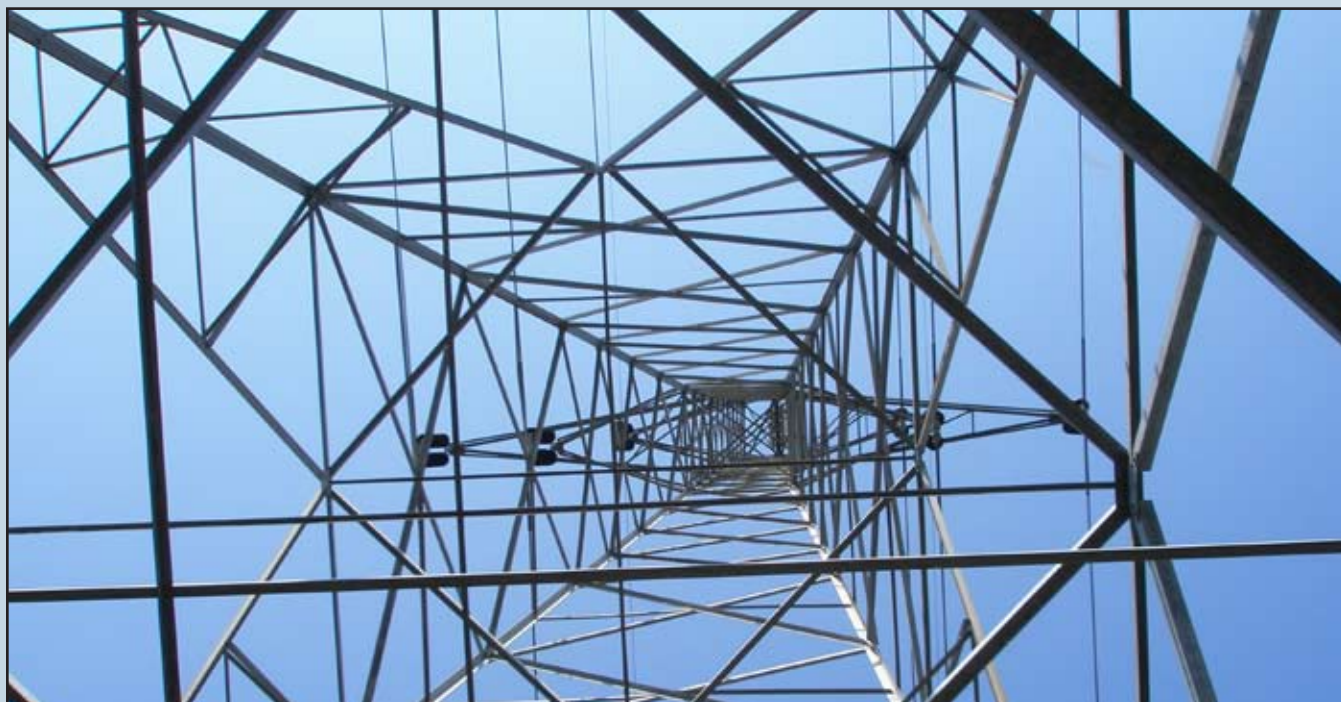
looking straight up from underneath the center of a typical lattice tower
