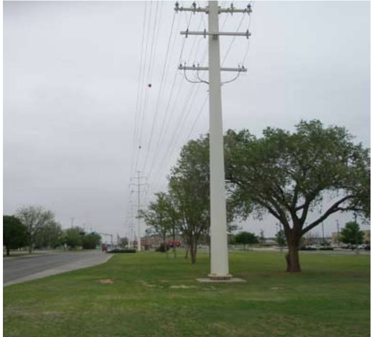
steel monopole that has been painted in Lubbock, Tx New Jersey only allows monopole structures painted to blend into scenery i.e. "pine tree green"
