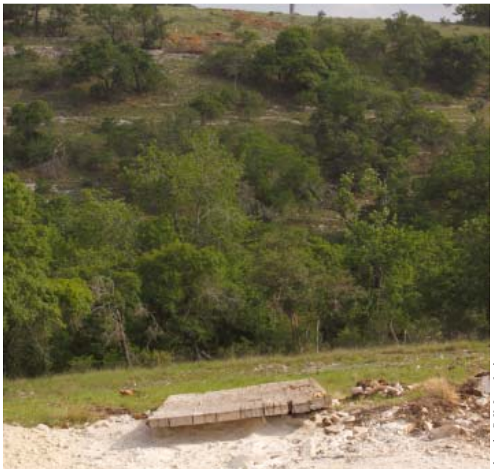
A large pallet covers a freshly dug hole awaiting a tower on a line Next Era Energy is completing. It runs from the world's largest wind farm near Abilene to Comfort in Kendall County.
